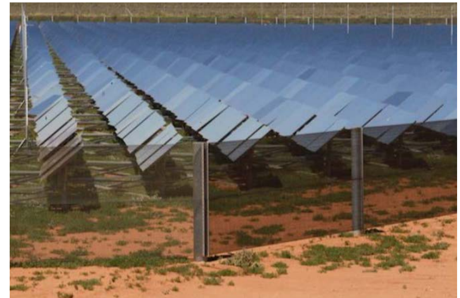
Figure. Wind fence surrounding utility-scale ground-mount solar PV installation
