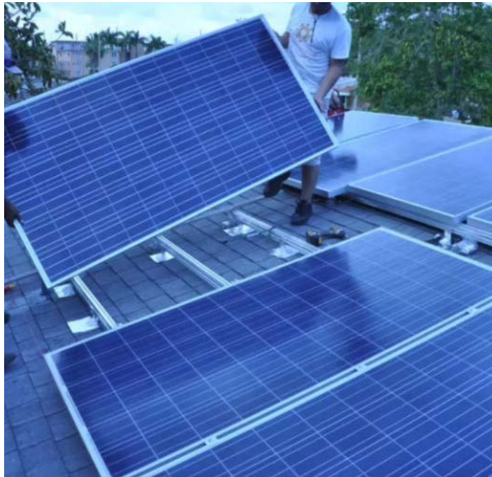
Figure. Three-framed rail system to support rooftop solar PV in hurricane-prone Florida
